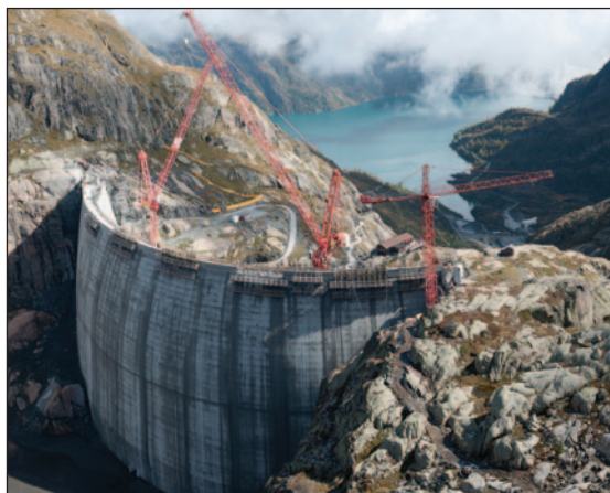
The construction works for the 20 m raising of the Vieux Emosson dam.
